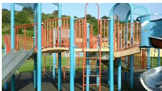
Image 3: Photograph of multiplay equipment at Whitehawk Senior, taken as part of the Annual Inspection
